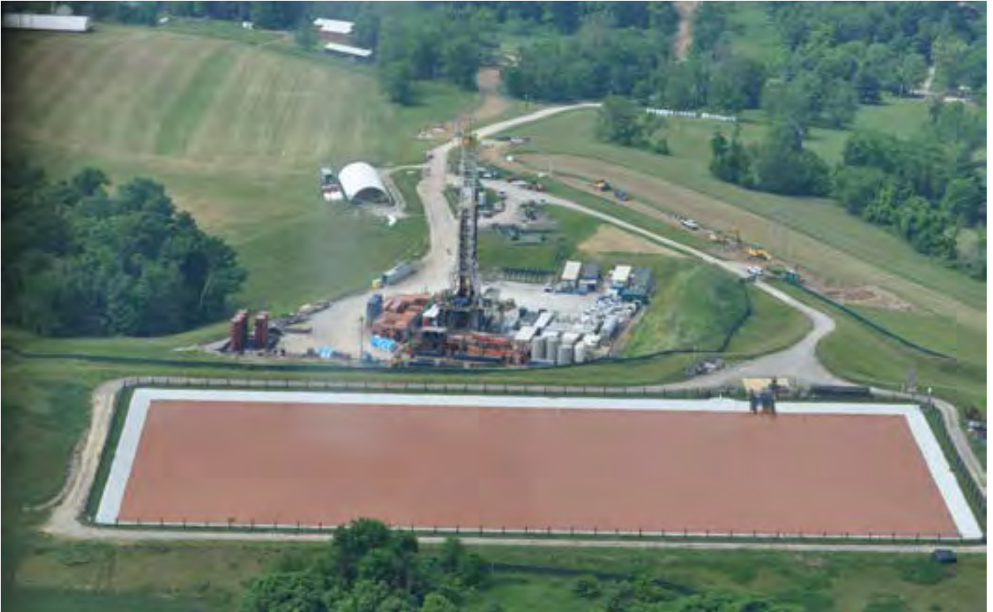
John Day unconventional gas well site and fluids impoundment in Amwell Township, Washington County, Pa., June 7, 2021. The Pennsylvania Department of Environmental Protection (DEP) cited discharges from this impoundment as some of the violations and releases that prompted the DEP's $4.15 million fine against Range mentioned on page 25 of this report. Photo credit: Courtesy of Marcellus Air.
