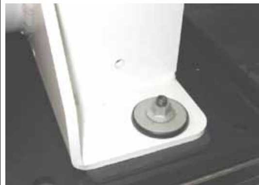
Figure 98. Tank isolator pad
